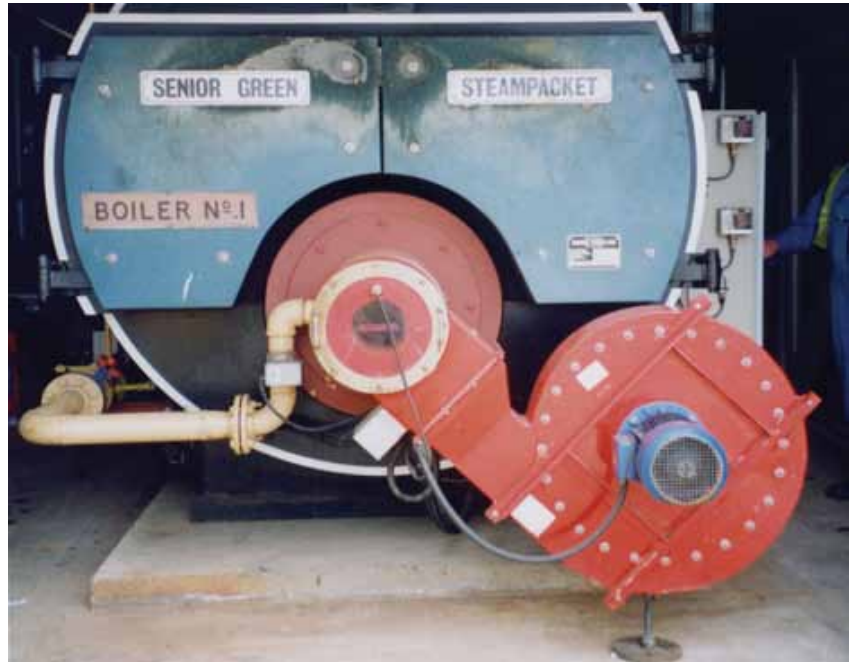
At Heinz, a well-placed yogurt pot made this boiler 16dB quieter
